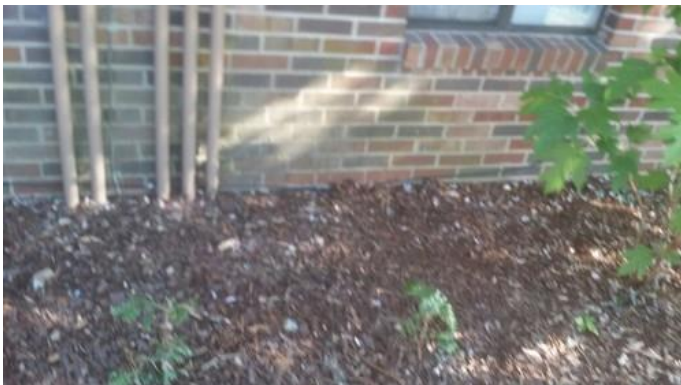
Low spots next to foundation, only mulch is present
