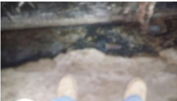
Water intrusion in crawl space
