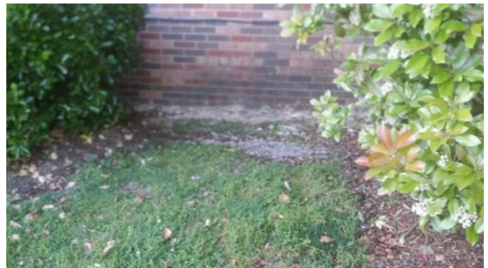
Low spot next to foundation
