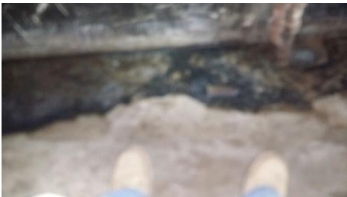
Water intrusion in crawl space
